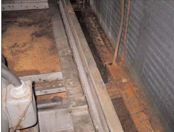
The condensate pan in this unit has been neglected for so long that it has rusted through.
